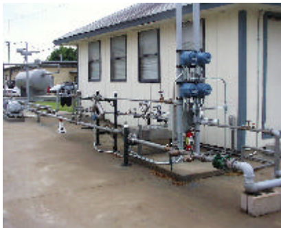
Hilly-Terrain Pipeline Meter Runs
